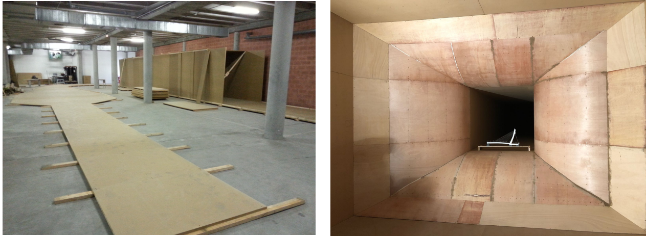
Figure 6. Construction of the wind tunnel in the EPM; construction of the basement on the left, the test section and the nozzle on the right.
